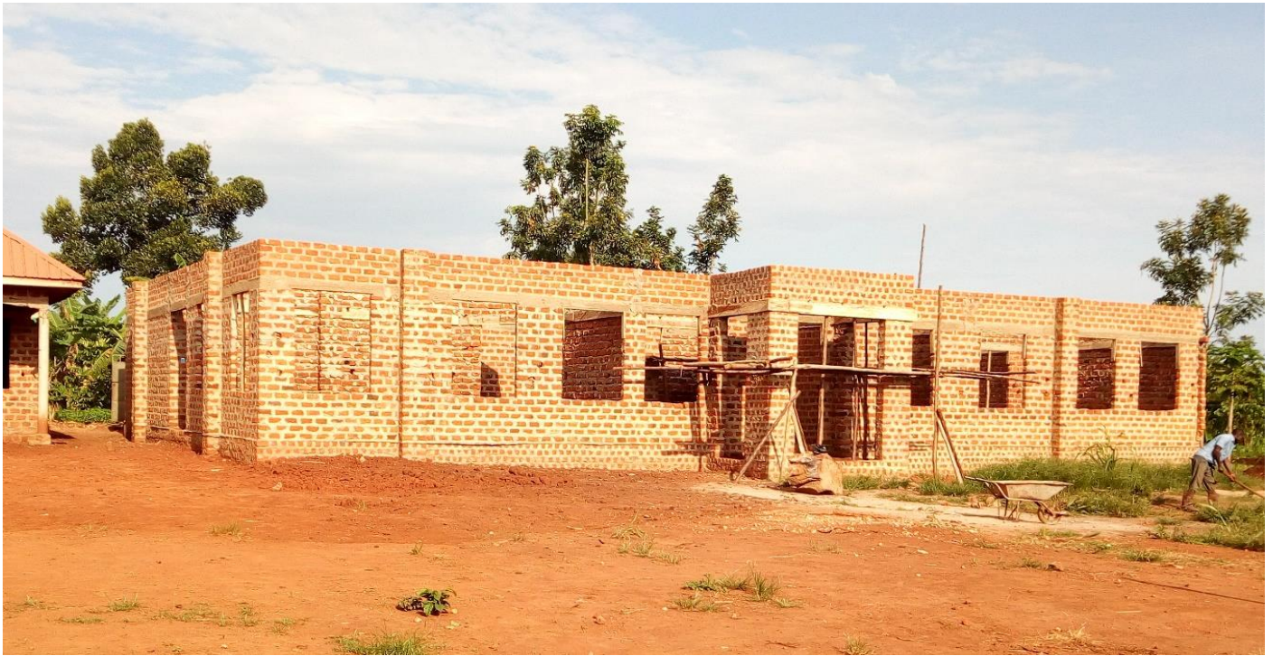
The current front view of the building just after completing walls and tie beam for the shade area
