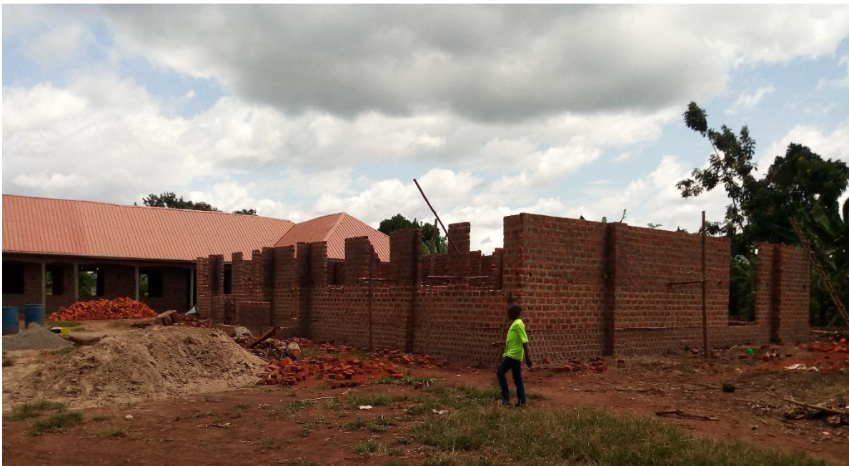
Look of the building at beam Level just before putting the tie beam and elevating the walls for the shade
